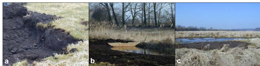
Fig. 2: Phase I of the rewetting; a. removal of drainage pipes; b. impounding ditches; c. leveling banks of ditches and small depressions
